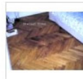
c. Paint stains in former studio.jpg
