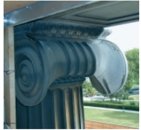
Examples of the work involved in cleaning and repairing the 1916 building, September 2000
